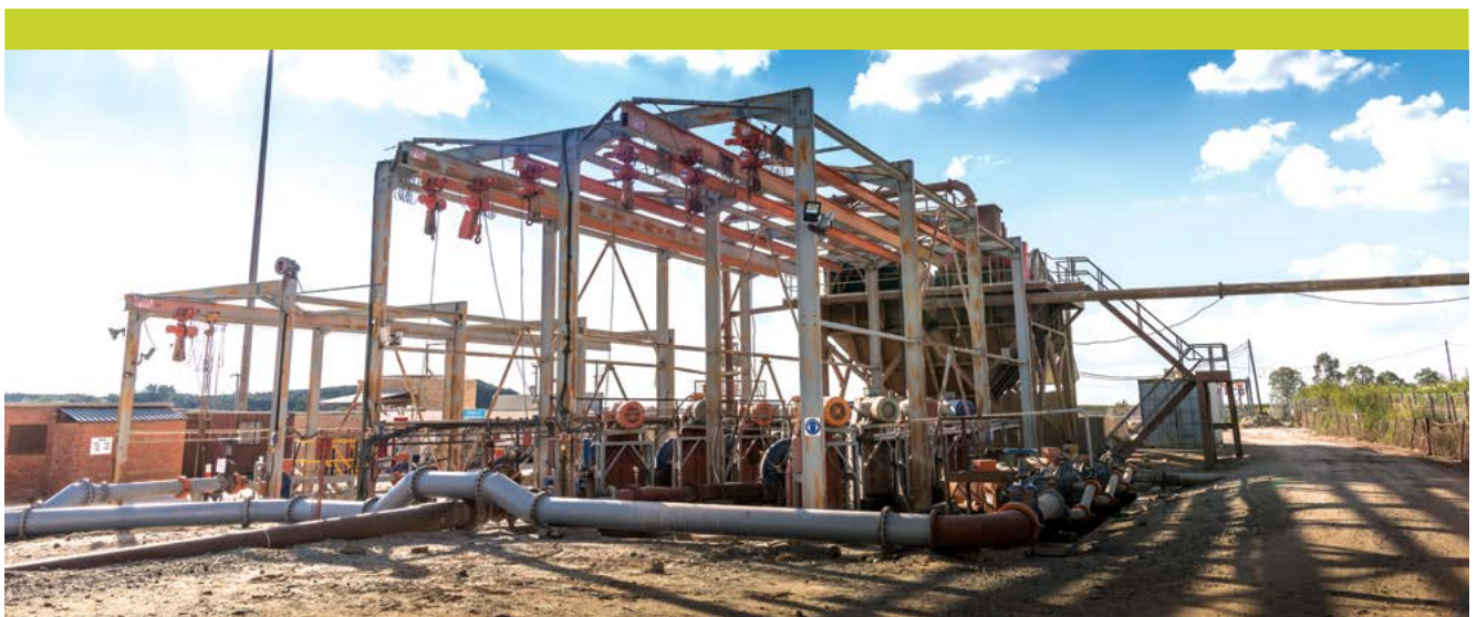
Saaiploas Plant residue pump station pumping to the St. Helena 1, 2 and 3 TSF
