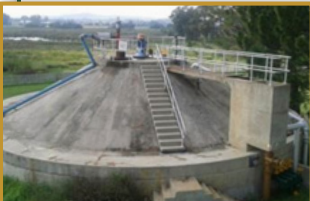
Anaerobic Digestion Reactor
